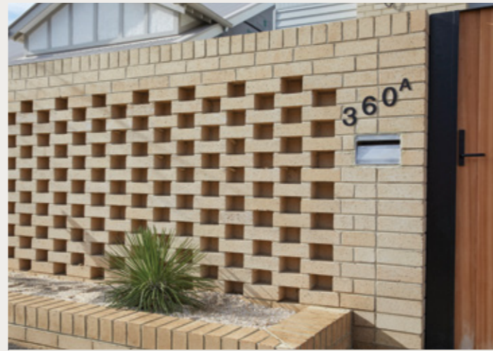
Jimmy & Tam's Brick Fencing. Organic White, Dry Pressed Architectural. Bond patterns: Soldier Course Headers / Stack Bond / Solid Brick Wall to Rear Leaf & Hit and Miss Brickwork. Mortar: Off-White. Joint: Round / Ironed.
